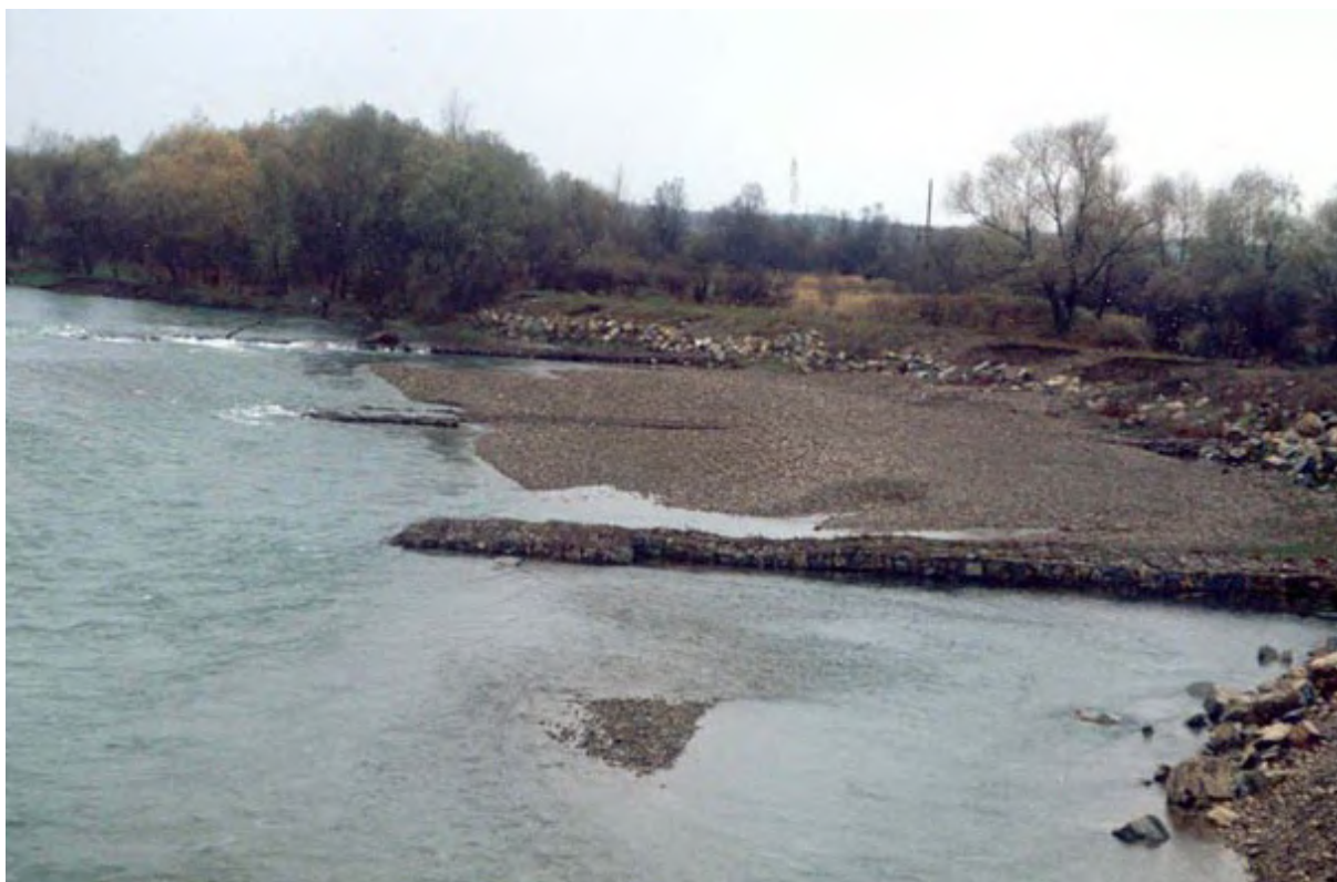
Figure 1. System of three groynes (gabion structures) to protect the base of the left bank of the Limnytsia River at the approach to the bridge and channel slope of the barrier dam on the Limnytsia River.
