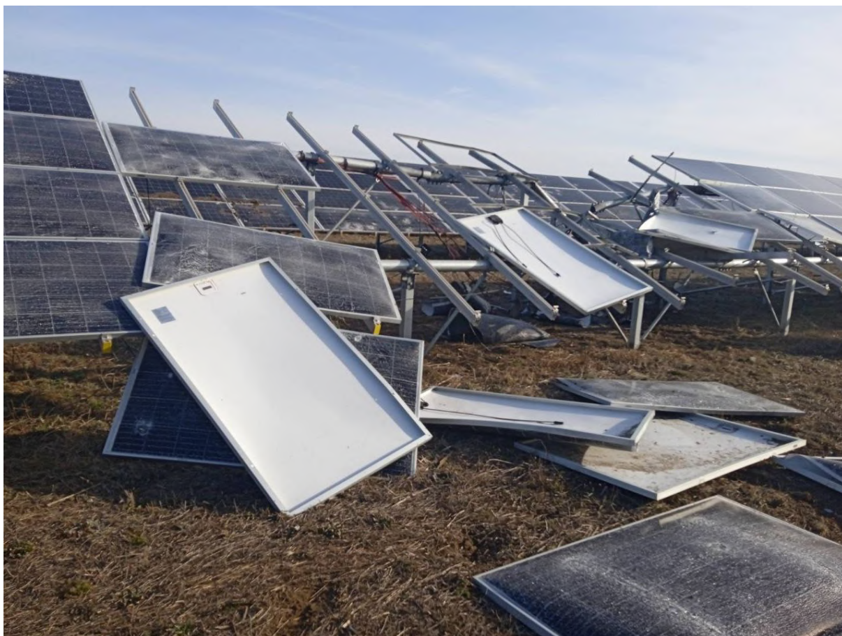
Figure 1. Damaged photo-voltaic power station.
