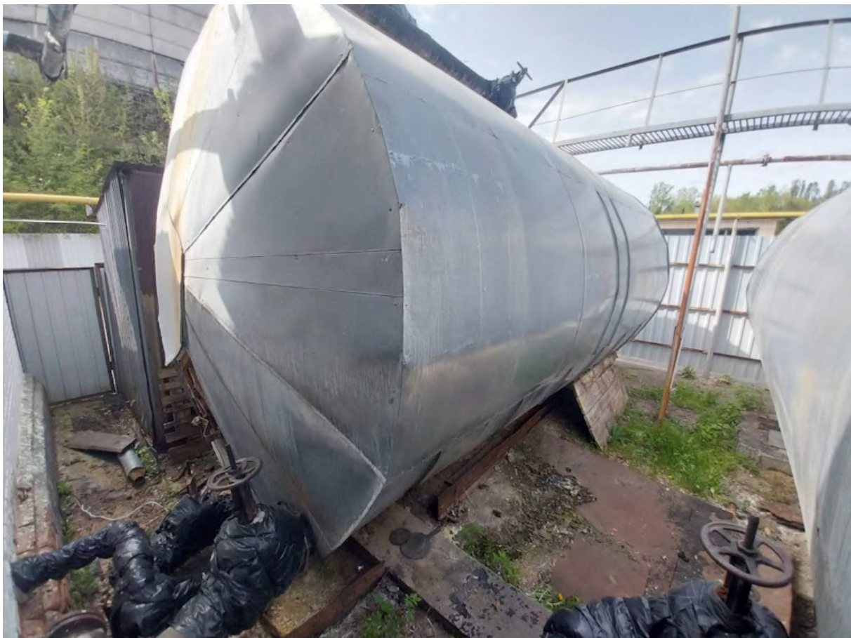
Figure 6. Storage capacity for a heating system with an estimated heat demand (thermal power) of 250 kW.
