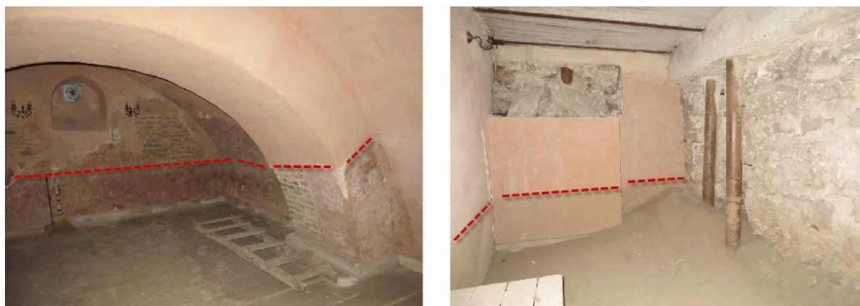
Figure 2. Traces of flooding and soaking in the basements (red line – flood level).
