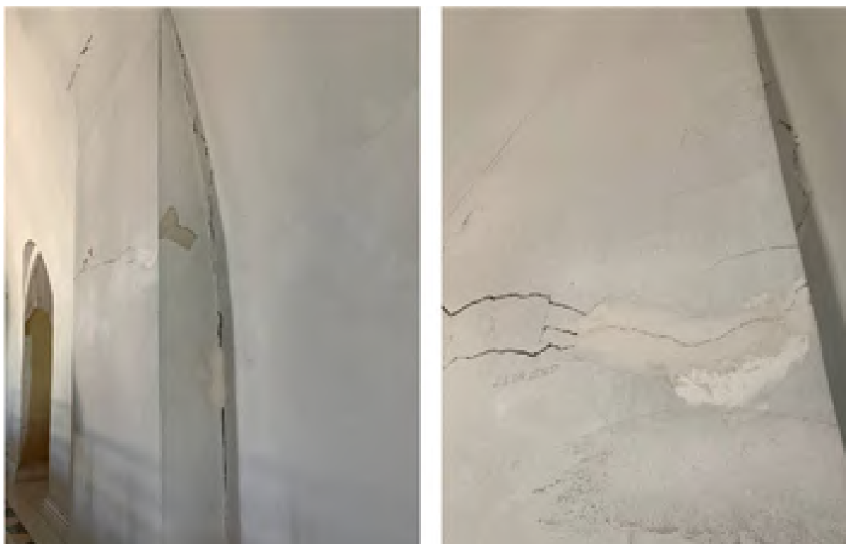
Figure 1. Structural cracks in the spalling of pilasters from the supporting (bearing) pillar, northwestern part of the 2nd tier (Preobrazhensky chapel).
