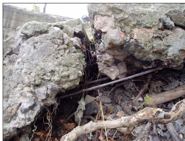
Fig. 3. Damaged area of the waterside protection.
