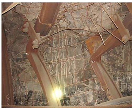
Fig. 6. Deformation of the frame stays.
