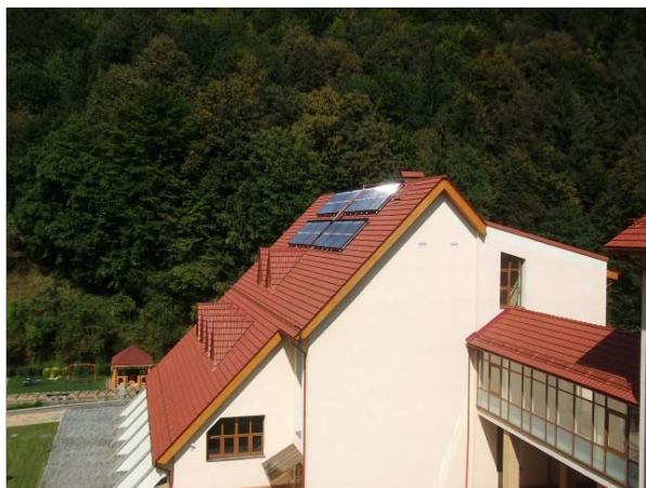
Fig. 3. Vacuum solar collectors are used to heat water in the sanatorium "Carpathian Stars", Yaremche.
