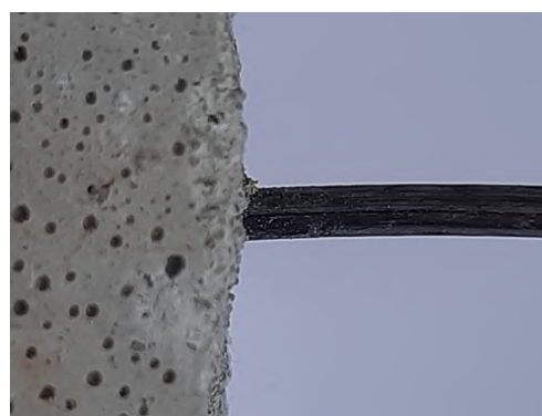
Fig. 12. Steel rebars embedded in plasticized AASC fine concrete mixed with seawater after 90 d of hardening (zoom x4) and based on sodium metasilicate.
