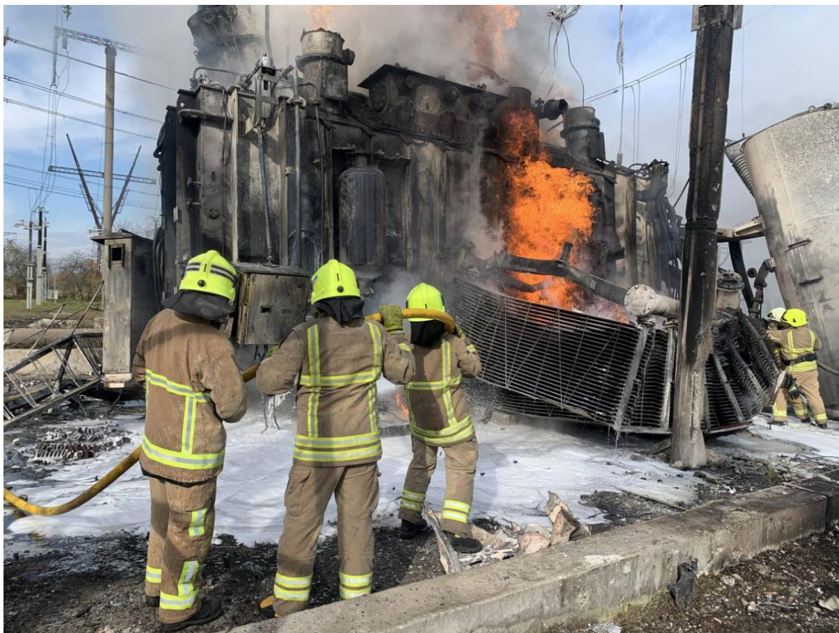
Figure 3. Power autotransformer destroyed by missile strike in Rivne region [8].
