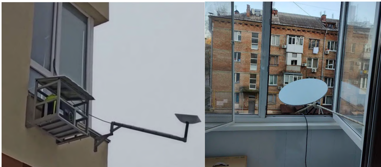
Figure 8. Examples of antenna installation of Starlink stations in cities of Ukraine (photo by https://highload.today ).
